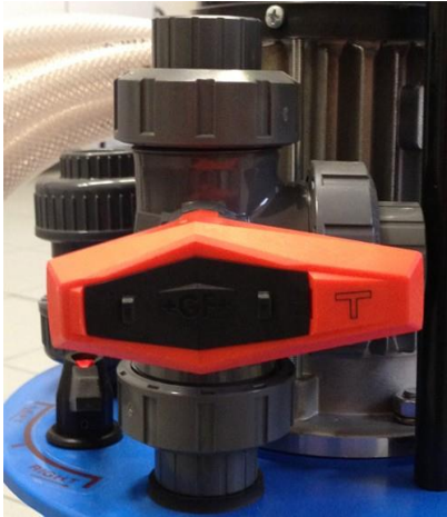
Valve in dump position
